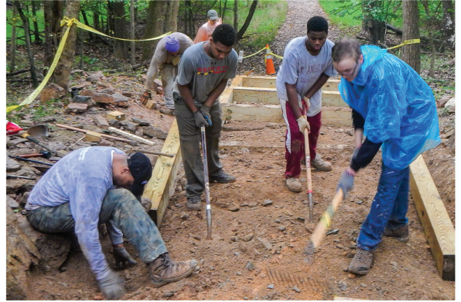
Eagle Scout Solomon Fenton (middle right) leads three volunteers on construction of the steps at Marsden Tract.
