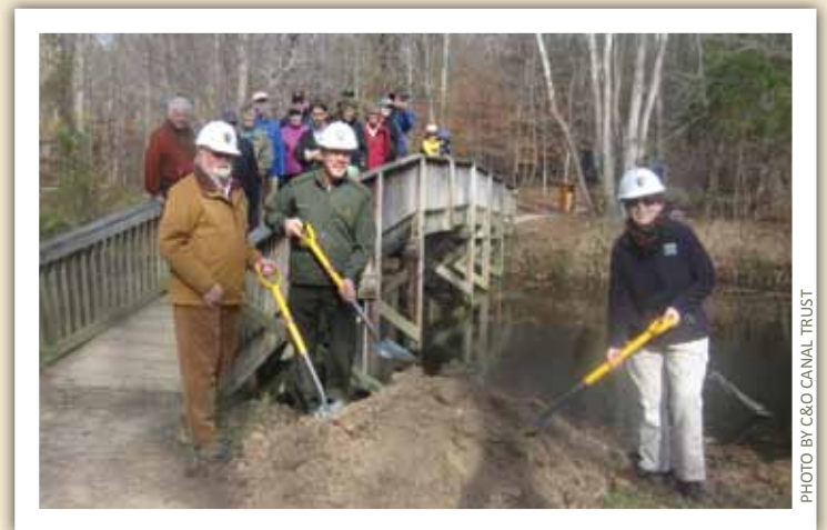
Board Chairman Mike Mitchell, Park Superintendent Kevin Brandt, and President Robin Zanotti break ground on the new bridge at Marsden Tract, while donors to the project look on from the old bridge.
